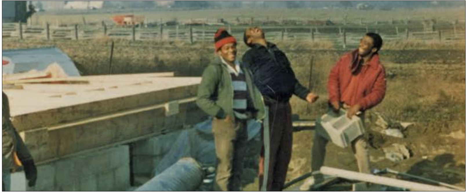
North Peel Community Church members can be seen working on church renovations in this photograph. The Peel Art Gallery, Museum and Archives is currently hosting an exhibition all about the church and its community. PAMA IMAGE
